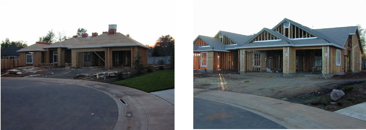
Figure 1. The pair of homes in Redding CA for demonstrating asphalt shingles with and without CRCMs.
