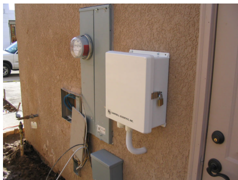
Fig. 1. Example of DAS, instrument wiring and electrical box for power meters.
