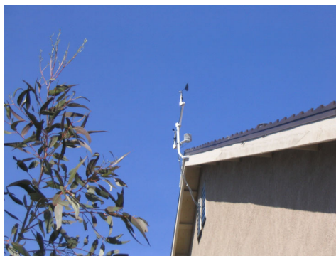
Fig. 2. Weather station installed 3-ft above ridge of C-style home.
